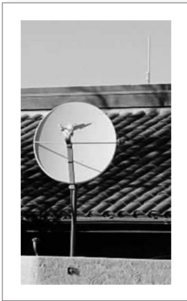
Figure 2: VSAT with WLAN monopole above flat roof
